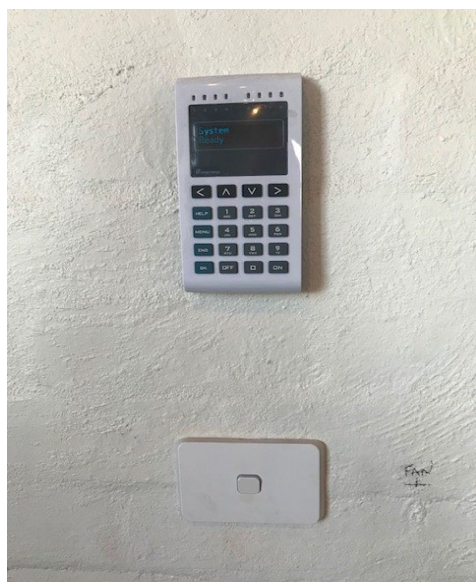
Boiler House can be disarmed and armed on this panel, or from the panels at the main theatre entrance, or office entrance. Doors must be closed when arming areas.
